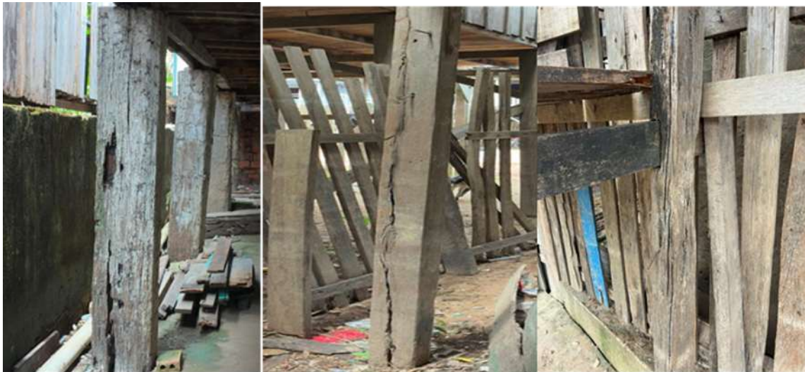
Fig. A10. Occurrence 10. Deep longitudinal cracks in pillars. GUT score: 36
