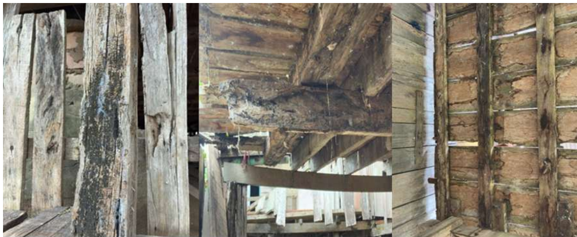
Fig. A1. Occurrence 1. Decay fungi in beams and pillars. GUT score: 125
