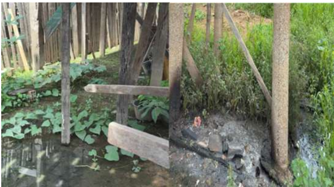
Fig. A8. Occurrence 8. Deterioration due to excessive moisture. GUT score: 80
