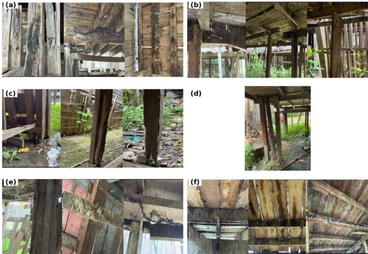
Fig. 3. Representative pathological manifestations documented in the evaluated stilt houses: (a) decay fungi in beams and pillars; (b) rupture/displacement in apparent structural elements; (c) degraded, hollow, or partially missing pillar bases and tops; (d) member instability; (e) visible subterranean termite tunnels; and (f) staining/mold fungi. Source: Authors (2026)
