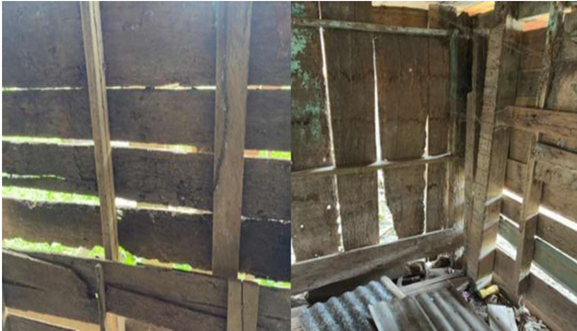
Fig. A9. Occurrence 9. Guardrails/enclosures with decay at the base. GUT score: 64
