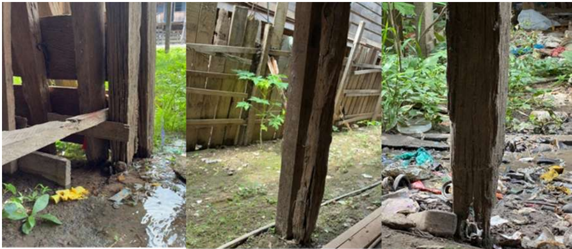
Fig. A3. Occurrence 3. Degraded, hollow, or partially missing pillar bases and tops. GUT score: 125
