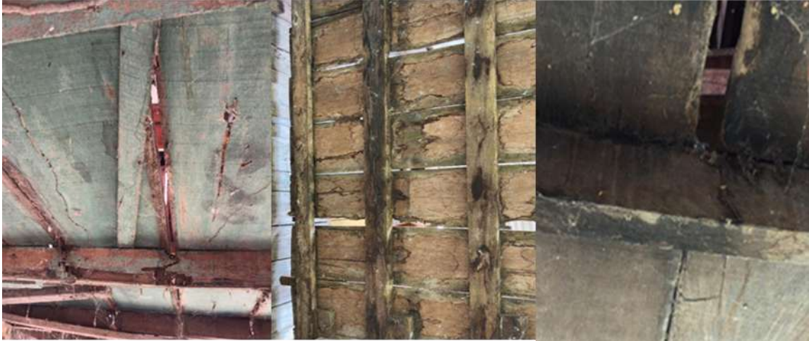
Fig. A11. Occurrence 11. Floor gaps larger than 5 mm. GUT score: 27
