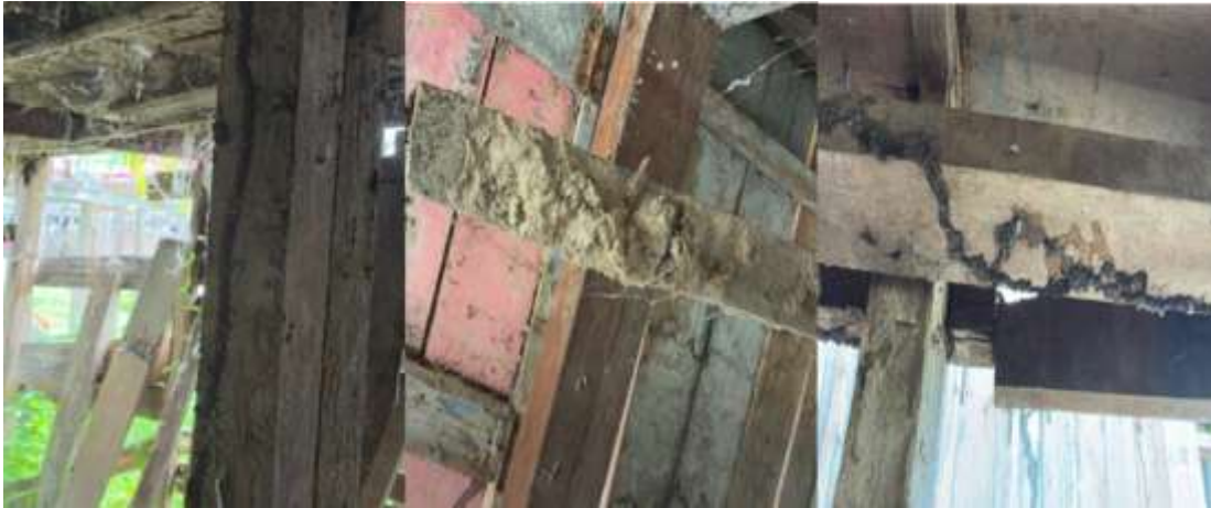
Fig. A6. Occurrence 6. Visible subterranean termite tunnels. GUT score: 80
