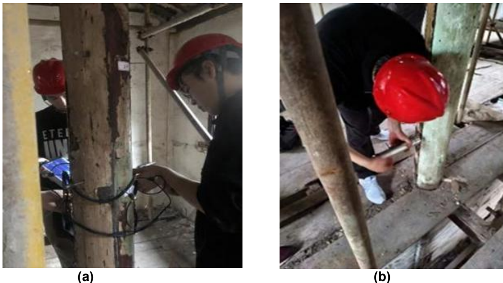
Fig. 3. (a) Sensor deployment site and (b) piro nail test site
