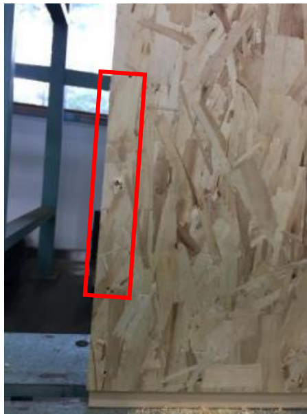
Fig. 8. The wood nails fractured and the shear panel separated from the stud
