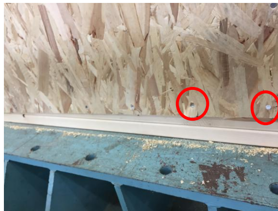
Fig. 10. The head caps of the twist nails dented in the shear wall connected by twist nails
